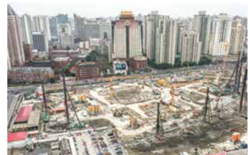
The construction site of ITC Phase 4 is progressing on schedule 徐家匯國貿中心四期地盤，工程進度理想
