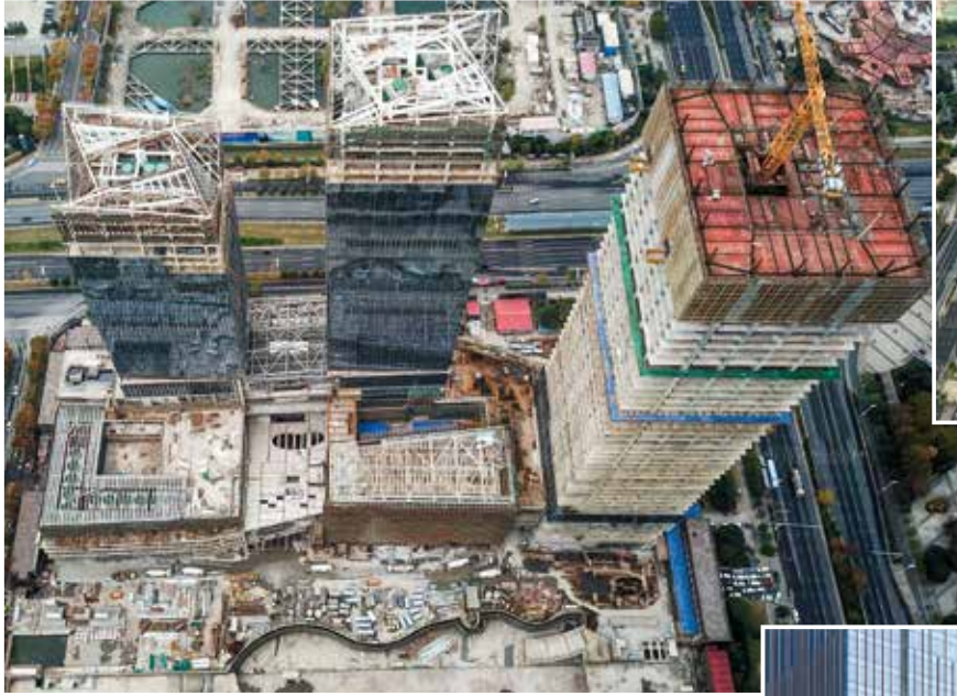
The first phase of the project will be completed by the end of 2018 (site photos taken on 30 November 2017)
