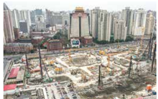
The construction site of ITC Phase 4 is progressing on schedule 徐家汇国贸中心四期地盘，工程进度理想
