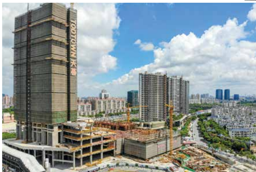
The facade is being installed on the Condos buildings (site photo taken in July 2018) 悦麓现正进行外墙工程 (2018年7月于项目实景拍摄)
