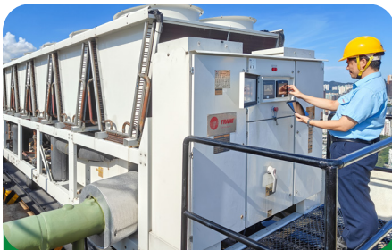
Retro-commissioning and chiller system optimization at Sun Hung Kai Centre
