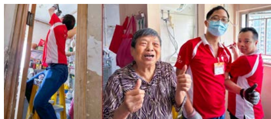
The SHKP Volunteer team utilizes their expertise to provide basic home-repair services for elderly households 集團義工隊運用自身專長，為長者家庭提供基本家居維修服務
