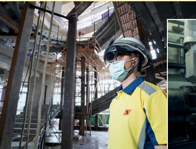
The construction team introduced mixed-reality technology, allowing construction to become more accurate and efficient
