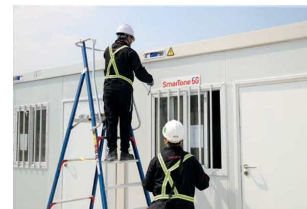
SmarTone built 5G networks at full speed for numerous sites where community isolation facilities and a hospital for emergency use are located. The photo shows antennas in the Tam Mi isolation facility, which provide a stable, high-speed 5G network for people admitted to or working in the facility.
