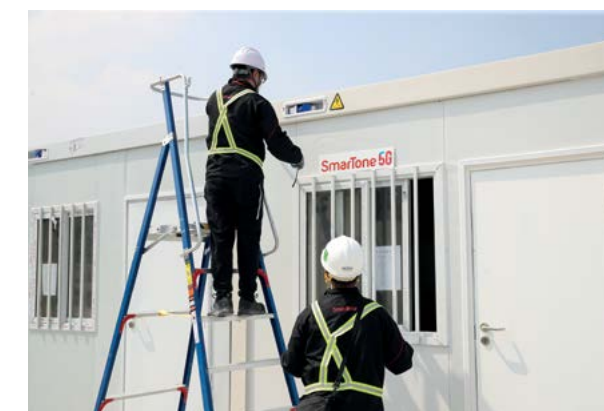
SmarTone built 5G networks at full speed for numerous sites where community isolation facilities and a hospital for emergency use are located. The photo shows antennas in the Tam Mi isolation facility, which provide a stable, high-speed 5G network for people admitted to or working in the facility SmarTone火速为多个隔离设施及应急医院搭建5G网络,图为SmarTone于潭尾隔离设施内的天线,为隔离人士及抗疫人员提供稳定及高速的5G覆盖
